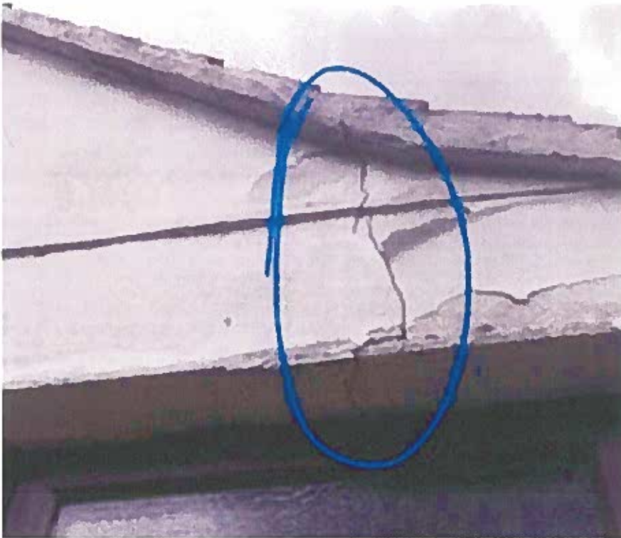
Image 8: Structural Crack over Window and up through roof verge pointing
