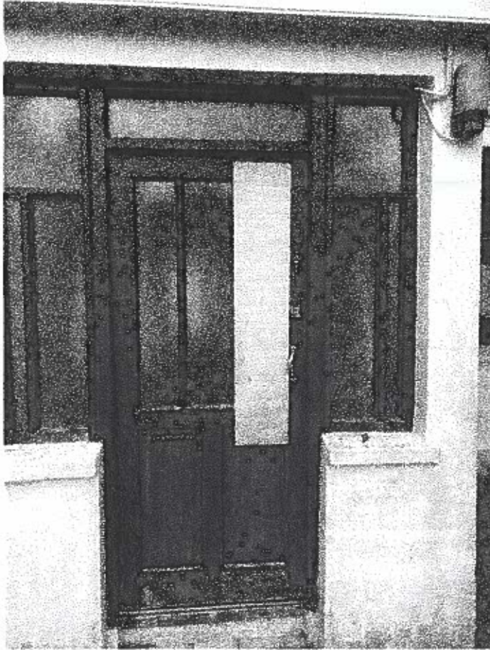
Image 10: Front Door in Poor State of Repair
