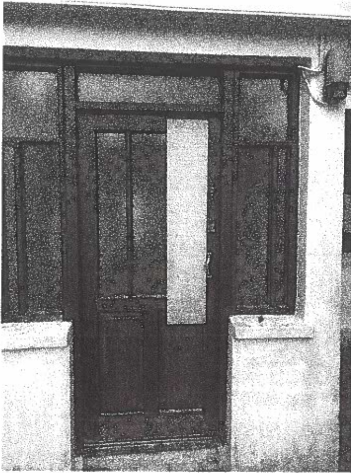
Image 10: Front Door in Poor State of Repair
