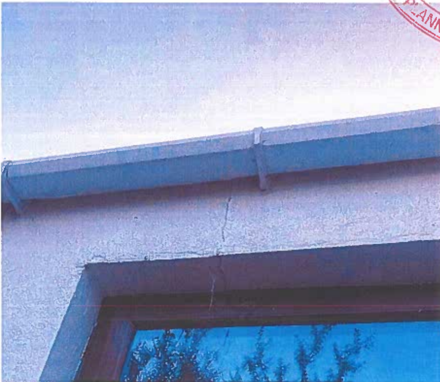
Image 9: Structural Crack over Window
