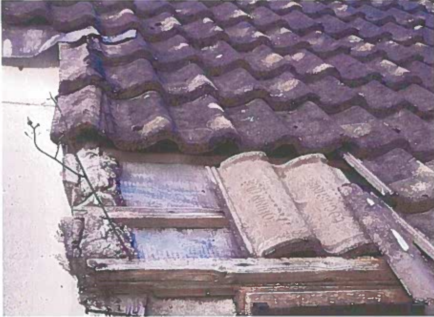
Image 6: Rotten Roof Timbers
