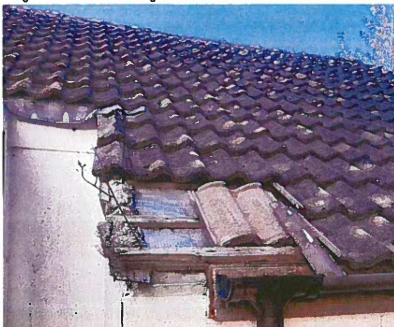
Image 5: Missing Roof Tiles, Rotten Rafters and Inadequate Gutters and Flashings
