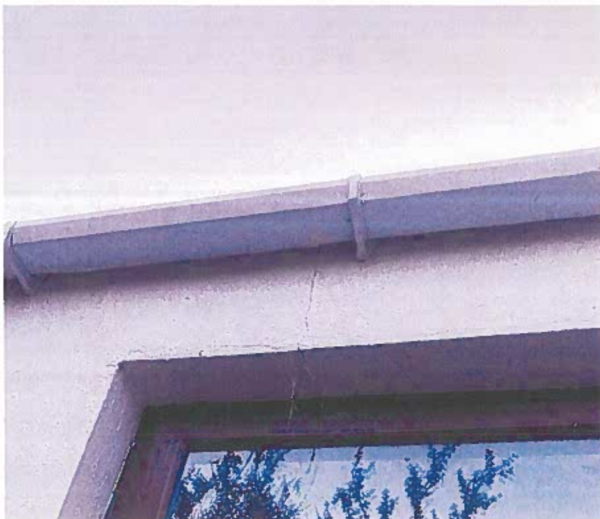
Image 9: Structural Crack over Window
