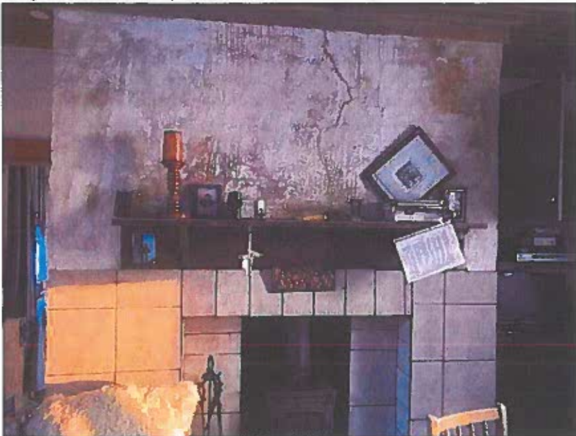
Image 3: Internal Dampness, Water-staining and Cracks on Chimney Breast
