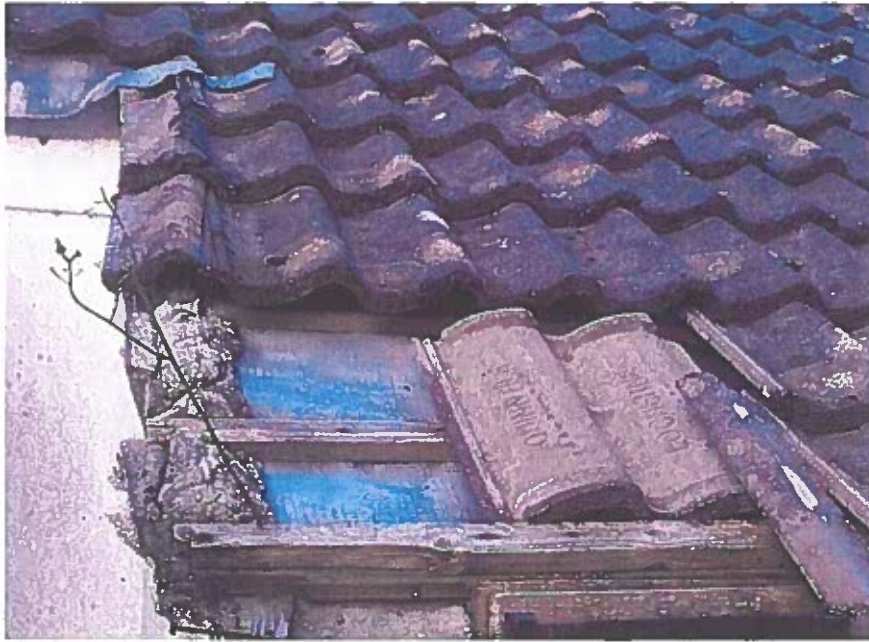
Image 6: Rotten Roof Timbers
