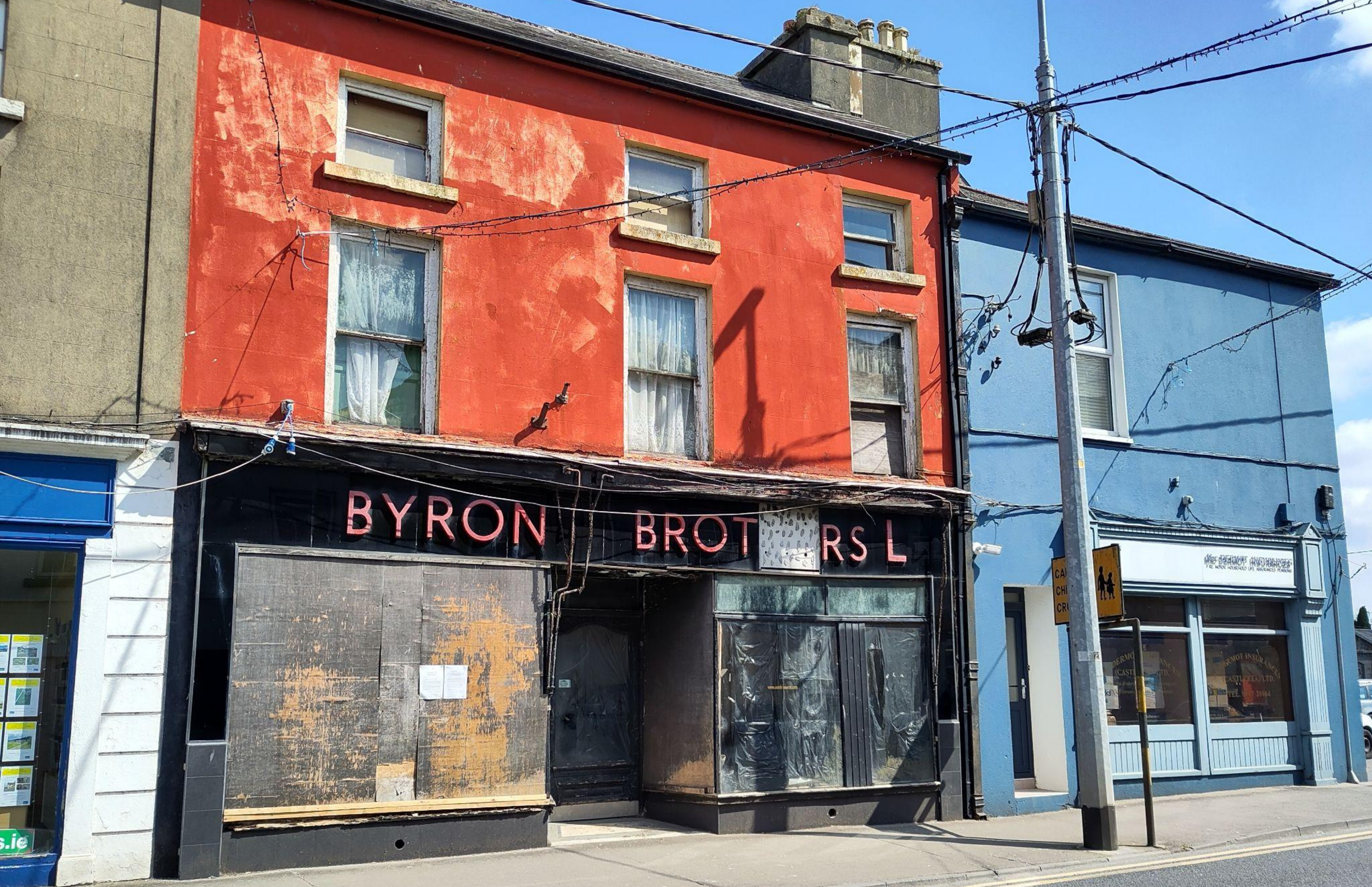
The vacant Byron Brothers building is a Protected Structure along Main Street falling into dilapidation
