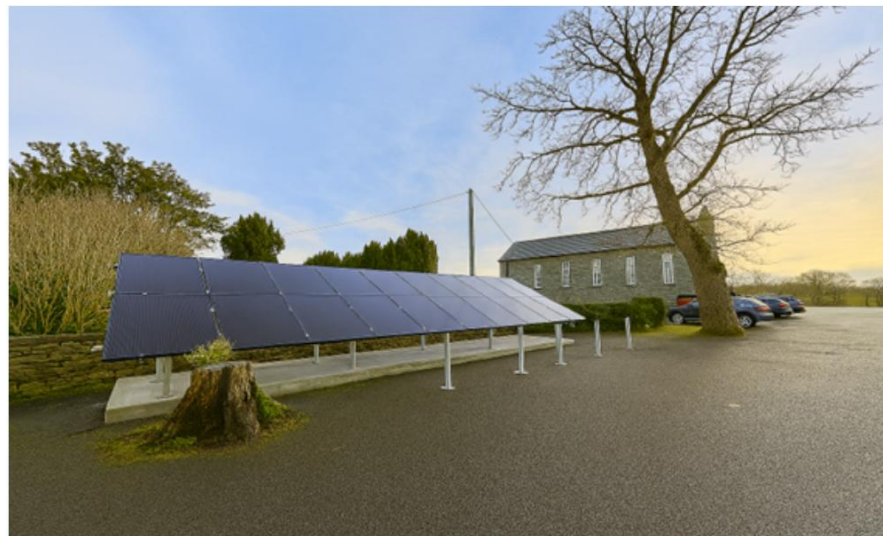
Field Trip: Roscommon Women's Network utilised Community Climate Action Programme funding to install solar panels and upgrade equipment, helping to reduce energy consumption and carbon emissions.
