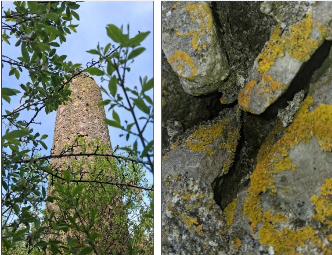
Plate 6-49. Representative images of Hodson's tower and examples of cracks within the stonework
