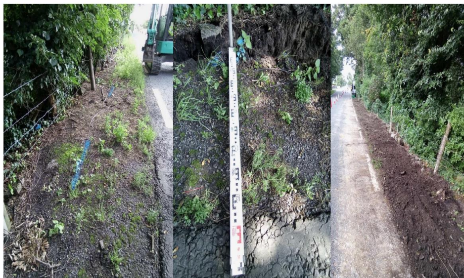
NBI verge excavation and reinstatement works above and all to minimum standards
