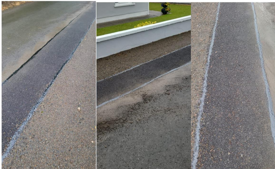
Example of NBI longitudinal trench reinstatement above that is of a high standard and meets the requirements of the Purple Book standards
