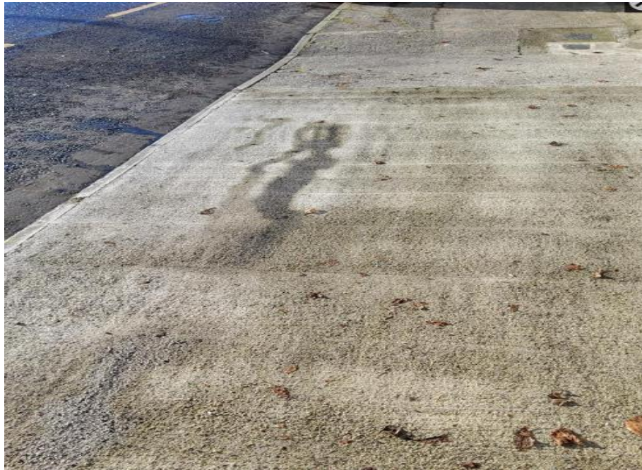
Image of substandard footpath reinstatement works above inspected and rejected by Roscommon County Council Engineer
