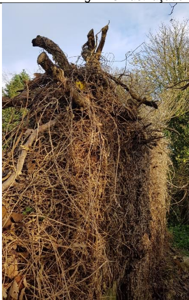
Fig. A44 Mature woody vegetation (branches recently cut back) on south gable of chapter room
