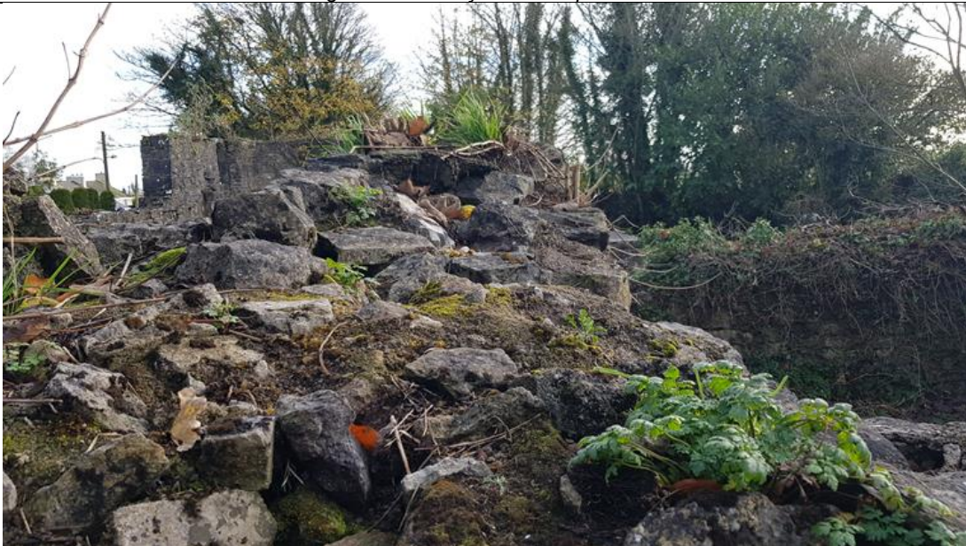
Fig. A47 Top of south external wall of nave, looking east towards apse (chapter room on left)
