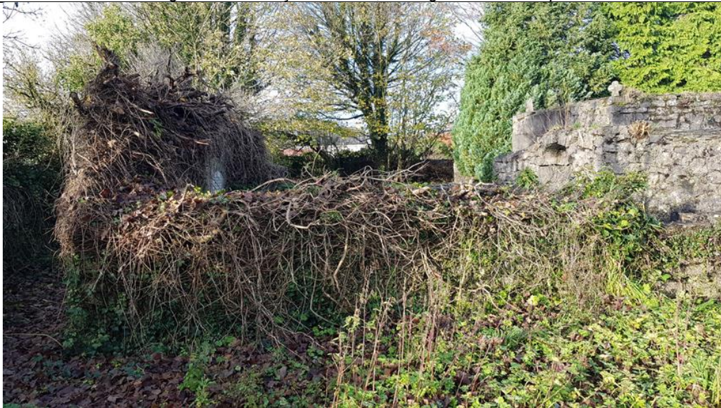
Fig. A43 East façade of chapter room, heavily overgrown with vegetation
