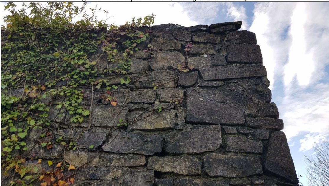
Fig. A34 Detail of north façade, with surviving window reveal (at north-east corner of nave)
