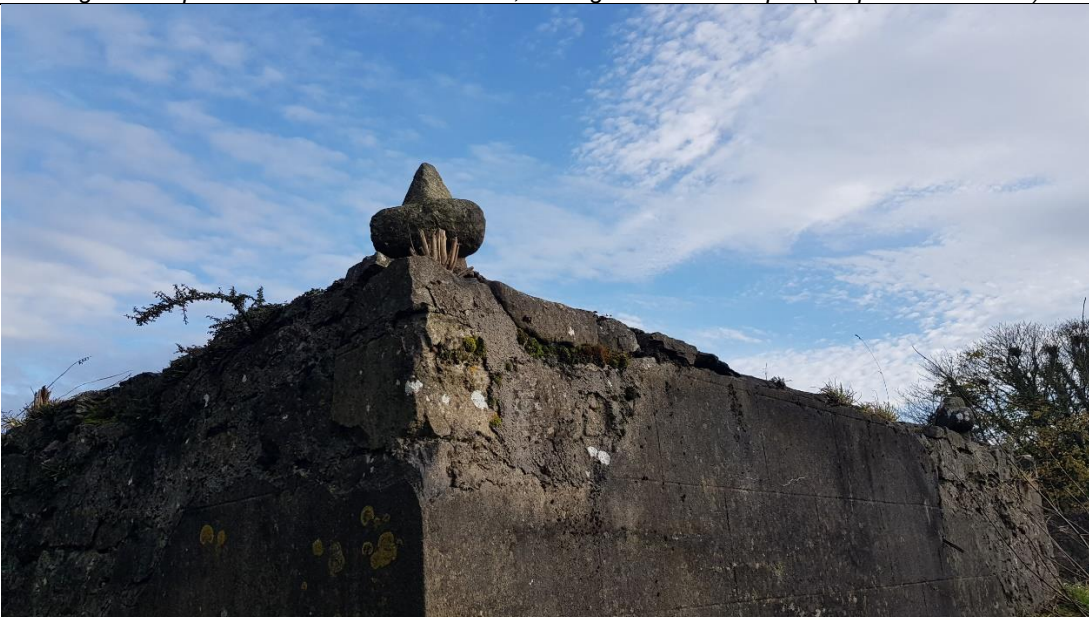
Fig. 48 South-west corner of tower, with lined and ruled external render, and relocated finials at corners
