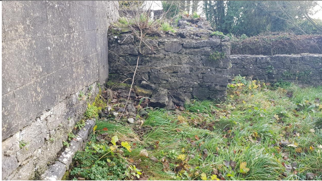
Fig. A49 Base of south façade of tower, looking east towards nave and chapter room
